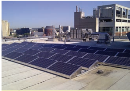
More solar panels will be added to these on the roof of the Northwest Tower of CHOP’s Main Building.
